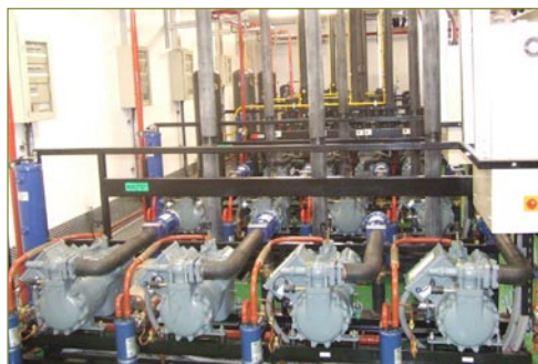
Bank of reciprocating compressors
