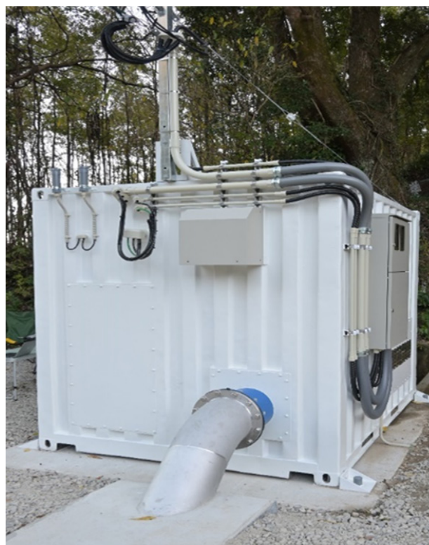
Figure 2. 10f container-based powerhouse of the Matsuguma SHP plant
