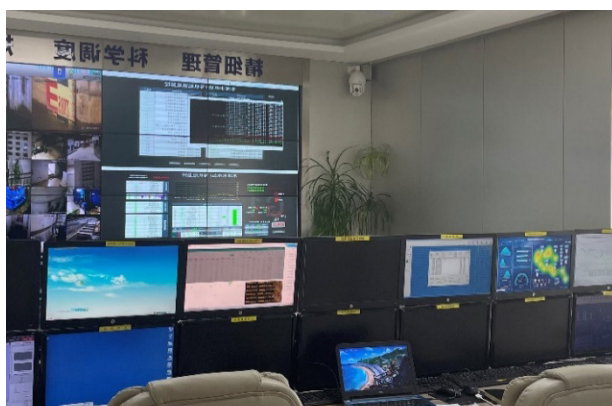
Figure 2. The Central Control Room
