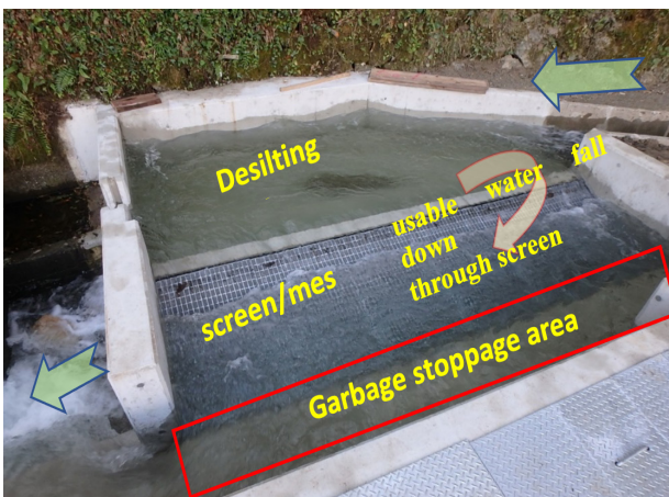
Figure 3. Forebay tank and desilting tank
