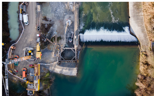
Figure 5. Excavation and Partial Removal of the Weir Structure for the New HSPP
