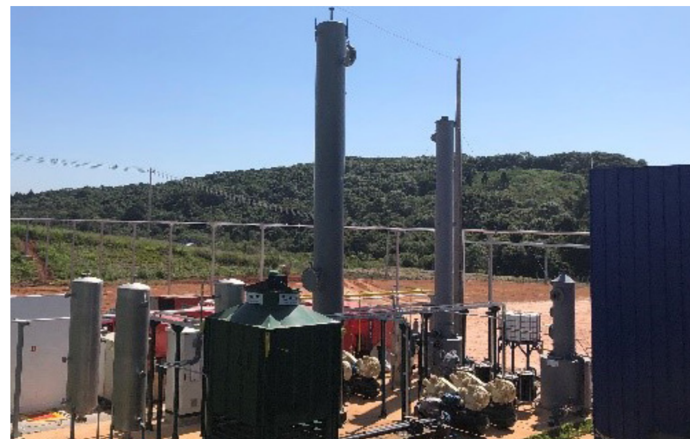
Biogas treatment plant in Brazil. (Source: Castrolanda)
